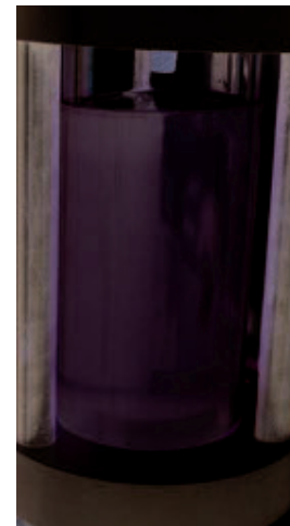
Fouled refrigerant, compressor faulty.
