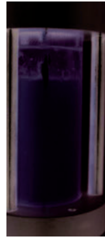
Insufficiently mixed oil and refrigerant.
